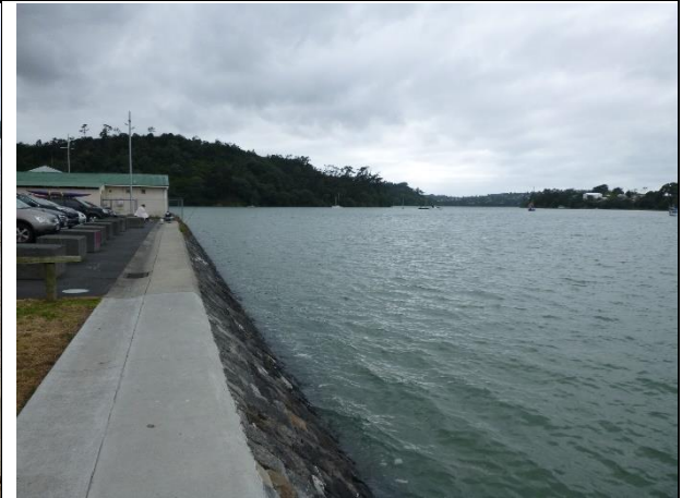
Photograph 6: Existing basalt seawall north of the proposed works area at high tide
