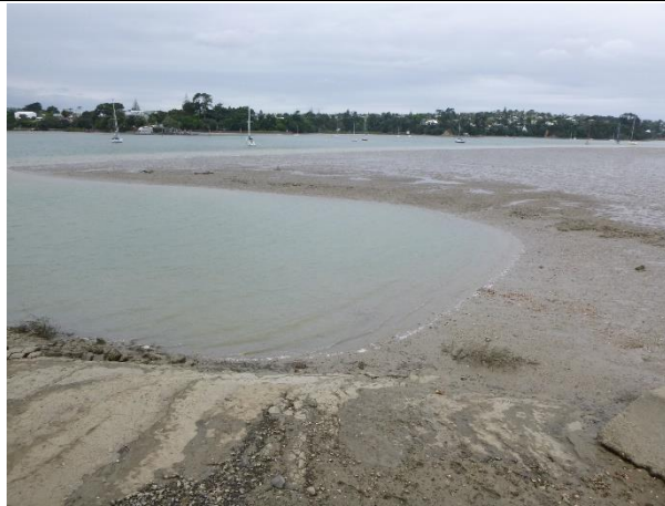
Photograph 5: Base of seawall facing toward dredged subtidal channel and proposed floating pontoon
